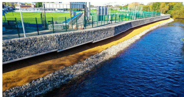
Dodder Greenway & Flood Defence Herbert Park to Donnybrook – cantilevering element & coco matting
