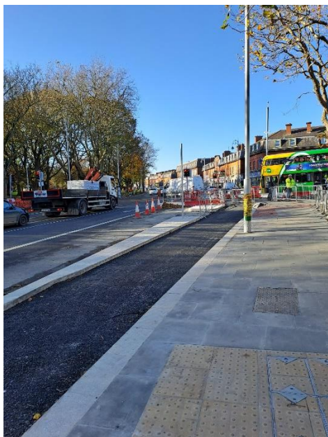
Clontarf to City Cycleway - Kerbing and paving works on the outbound side of the Clontarf to City centre Scheme
